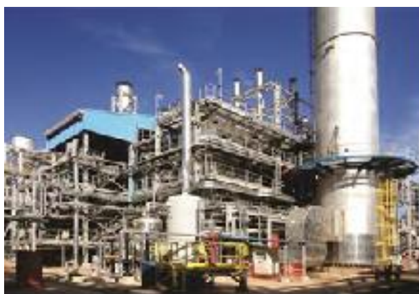
Chart 8: Oil & gas fired boiler
