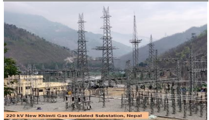
Exhibit 4: Largest GIS substation executed in Nepal
