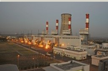
Uno-Sugen Plant (382.5MW), Surat, Gujarat
