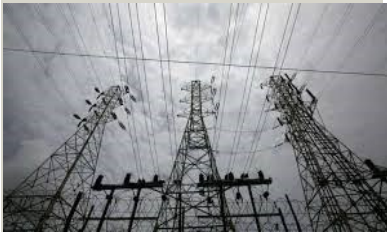
Power distribution lines
