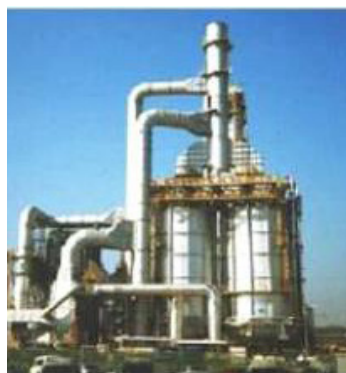
Crude Distillation Unit (CDU) Heaters
