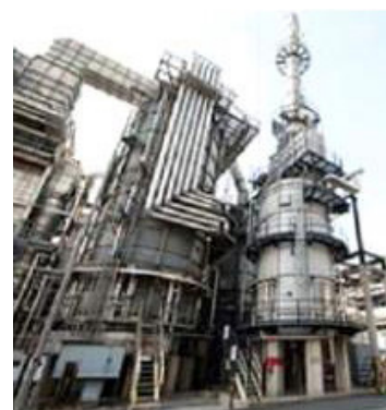
Hydro-treater/HDS Heaters, Hydro Cracker Heaters
