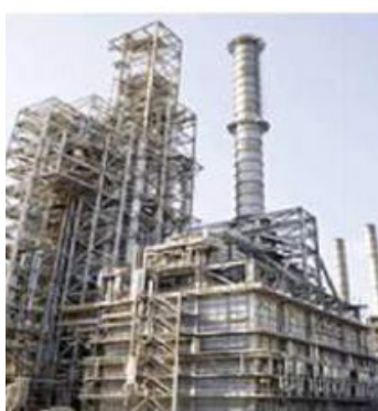
Catalytic Reforming Heaters
