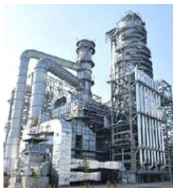
Vacuum Distillation Unit (VDU) Heaters
